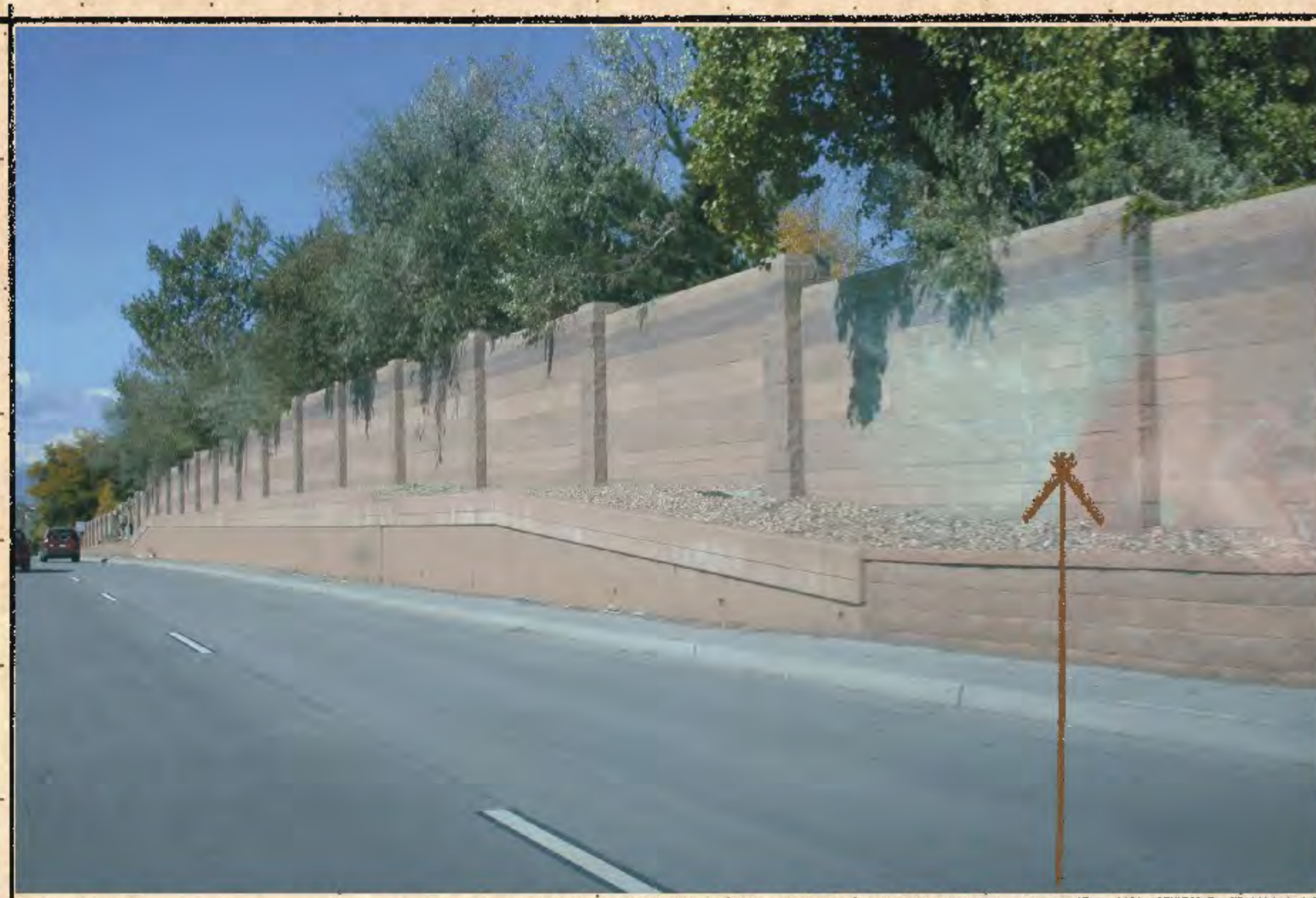
Tall masonry noise barrier wall along a limited access highway, consisting of concrete block with bands of different colors. If it is absolutely necessary to have a tall wall for sound attenuation then this is one of the more effective examples. Pilasters and banded colors add interest. Coarse textured surfaces help reduce noise reflection. Some shrub planting along the face of this wall would soften its appearance as well as intercepting dust. Note there is no sidewalk or landscape strip on this roadside which gives the otherwise attractive wall a somewhat harsh look.
